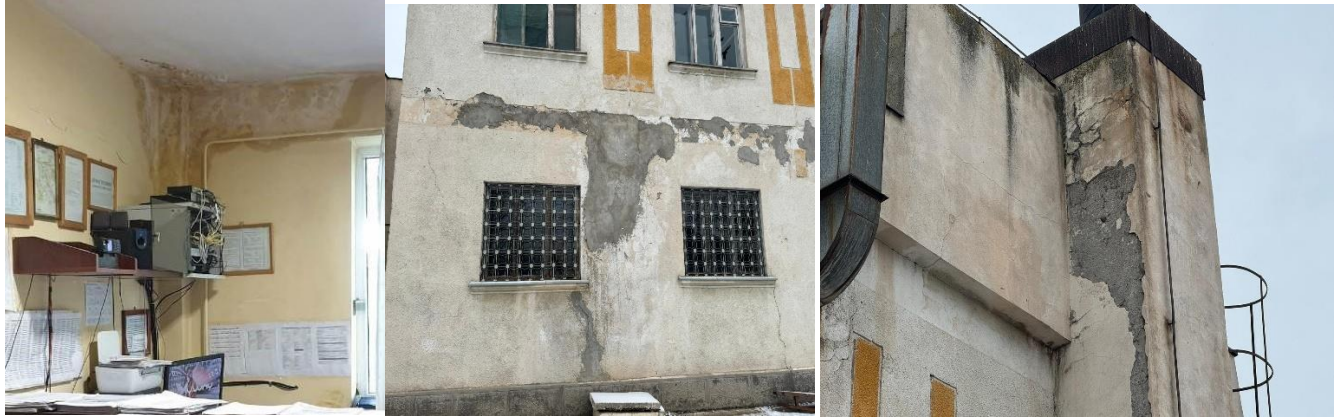
Figure 7 Visible deterioration of the existing ZFD's buildings
